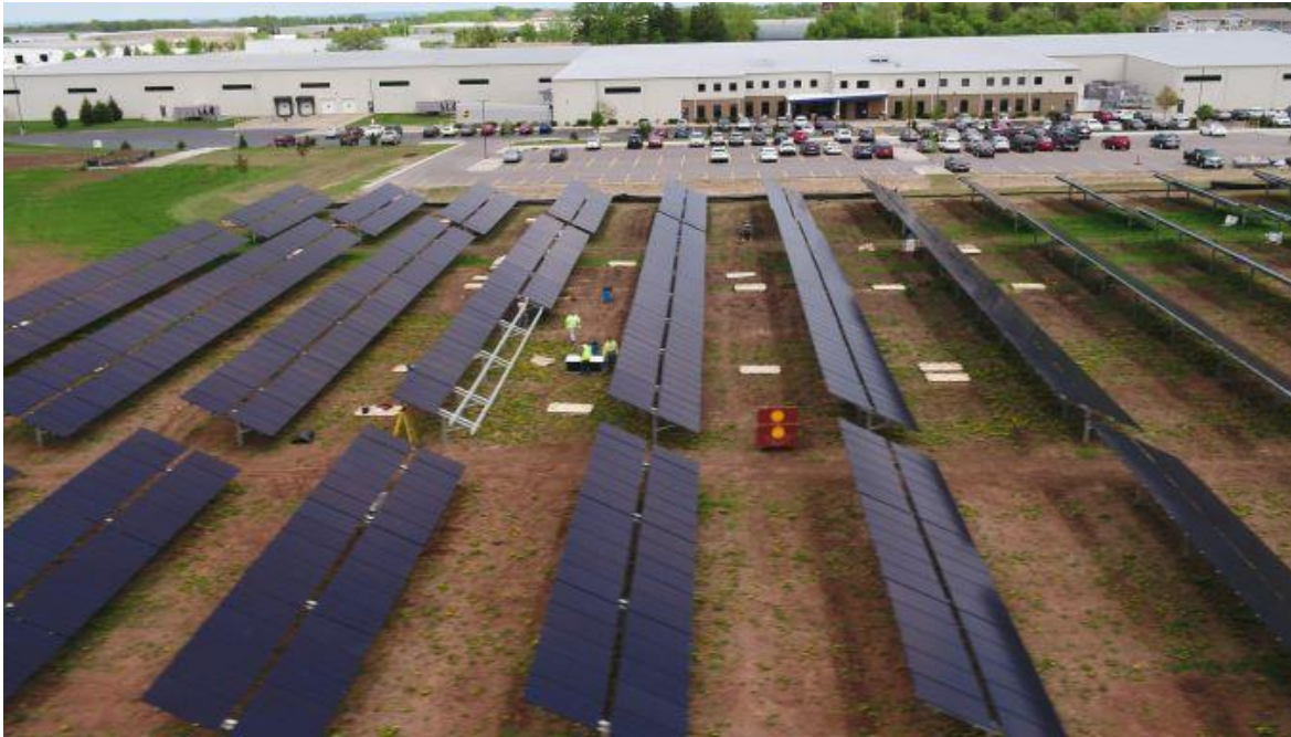
Installation of Oshkosh Distribution Center (DC) solar array. Photo looks eastward towards the DC building
